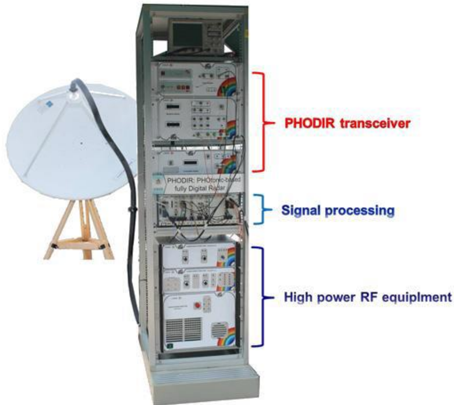
Figure 6 General view of the entire device [6].
